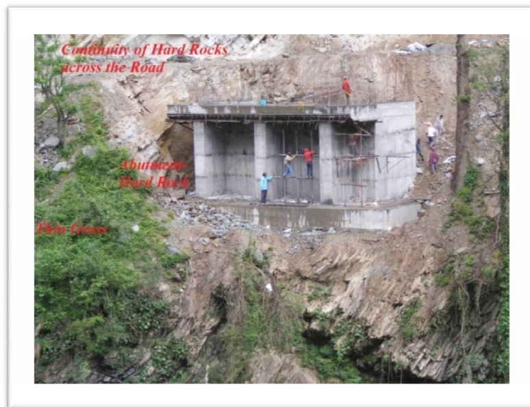
Picture 1 Field Photograph of the raft foundation on Srinagar side, Pannar Bridge
